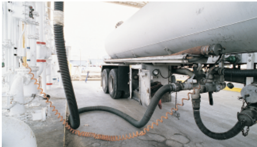
FIGURE 21–12 The ground wire on a fuel truck prevents explosion of the gasoline vapors.
